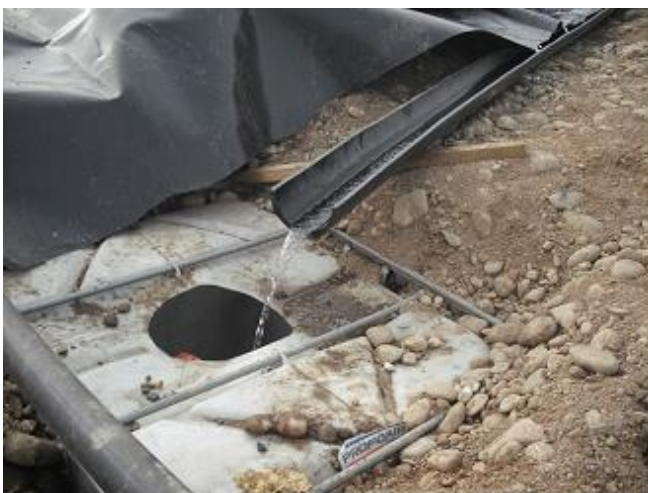
Figure 9. Drained water collection.
